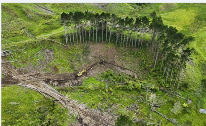
Felling the final trees from Ture Matai Reha pa site with the armoured log extraction corridor.
